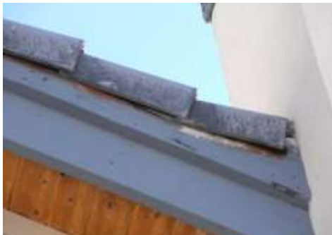
Roofing tile lifting
