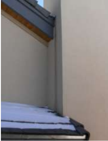
EIFS Façade – potential water damage
