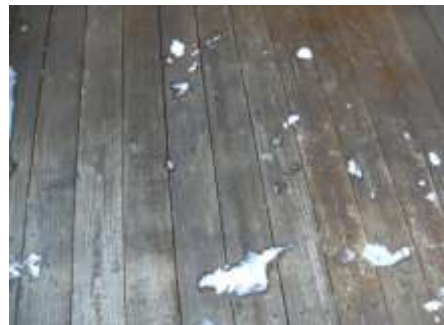
Decking stain faded
