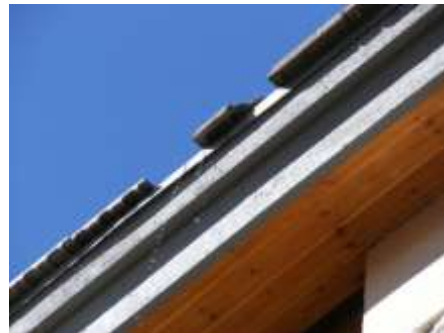
Roofing tile missing
