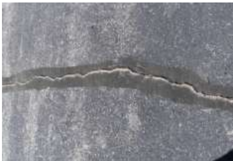
Asphalt expansion crack
